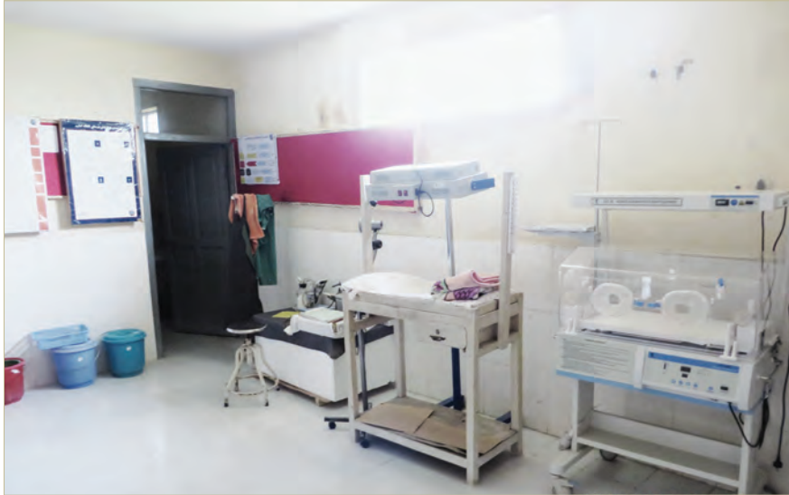
Maternity-ward equipment at Health Facility 307, Nangarhar Province. (SIGAR photo)
