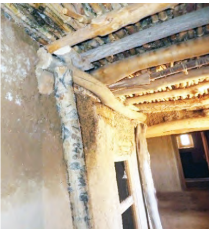
Leaking roof and saturated walls at a health facility in Ghazni Province. (SIGAR photo)
