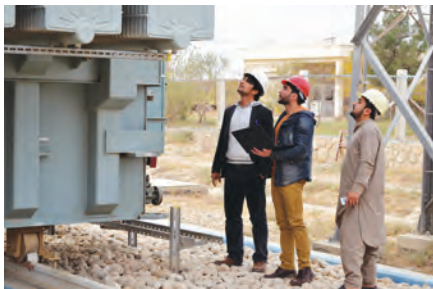
Trainees in the Power Transmission Expansion and Connectivity Project in Mazar-e Sharif learn about asset management and maintenance. (USAID photo)
