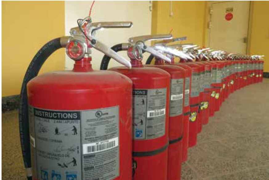
Fake-label fire extinguishers with identical serial numbers were discovered during a SIGAR inspection of a women's dorm in Herat. (SIGAR photo)
