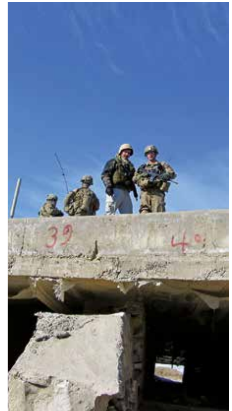
A SIGAR investigator traveling with U.S. military personnel confirmed that anti-terrorist gratings had been falsely reported as installed at this highway culvert. A court proceeding related to the fraud was conducted in July 2017. (SIGAR photo)
