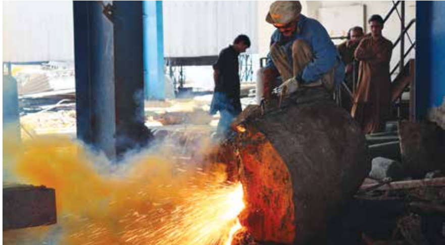
A welder at Maisam Steel Mill , an enterprise established with aid from USAID's Assistance in Building Afghanistan by Developing Enterprises Program. (ABADE photo by Sulaiman Latifi)
