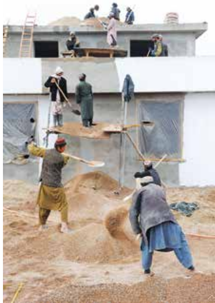
Workers move gravel up to the roof of a new prison in Uruzgan Province, 2011. (USAF photo by 1st Lt. Matt Schroff)
