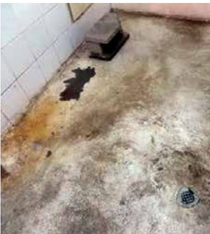
Improperly sloped shower floor with mold in one officers' barracks. (SIGAR photo)
