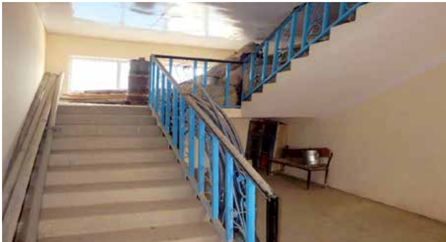
A suboptimal staircase installation in Baghlan Province. (SIGAR photo)
